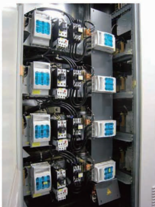
无源滤波设备 Tuned filter circuits equipment
